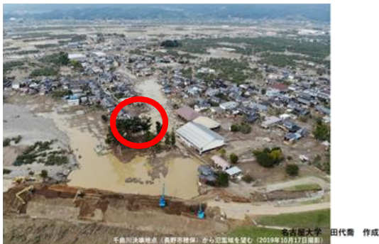
図1 穂保地区の千曲川決壊と復旧作業の様子 Fig.1 Chikumagawa River embankment collapsed and restoration work in Hoyasu district.
