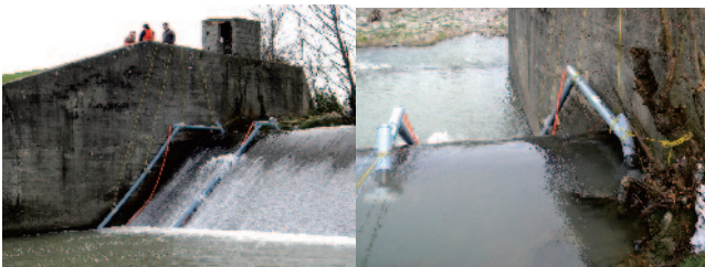
Fig.12 Fishway No.1 and No.2 installed at Pasikhan Dam in Gilan Province. Fishway No.1 is fixed to trees with chains, and fishway No.2 is fixed to the wall with ropes.
