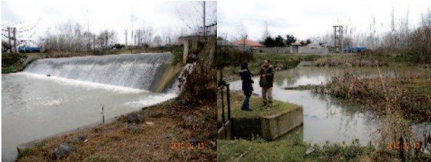
Fig.5 One of the typical weir in Giran Province. The left is the downstream side and has a slope. The right is the upstream side and a water gate can be seen on the left bank.
