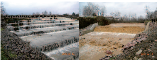
Fig.6 Steps and slopes on weirs in Giran Province. Small-step type and multi-slope type weirs are probably traditional design methods in Giran Province.
